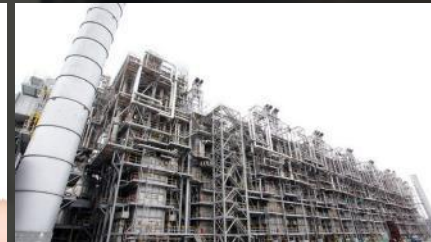
Petrochemical plant Insulant
